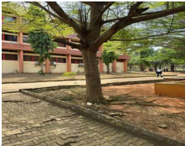
Plate 11: Tree root uplift displacing and fracturing interlocking paving blocks — trip hazard on active pedestrian route
