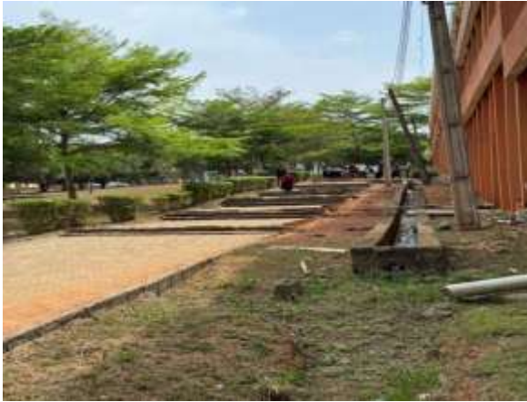
Plate 8: Stepped path beside academic block — stagnant drainage channel, eroded steps, debris
