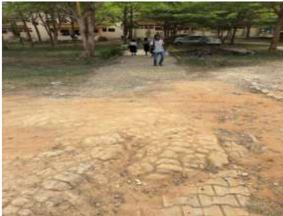
Plate 12: Severe paving degradation — blocks buried under laterite, pedestrians on bare soil surface
