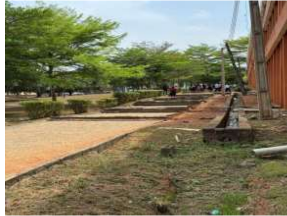
Plate 9: Same route from above — paving intact (left) but drainage channel collapsed (right), pedestrians in use
