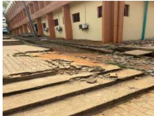
Plate 13: Complete paving collapse beside academic building — broken blocks, exposed subbase, crumbling steps
