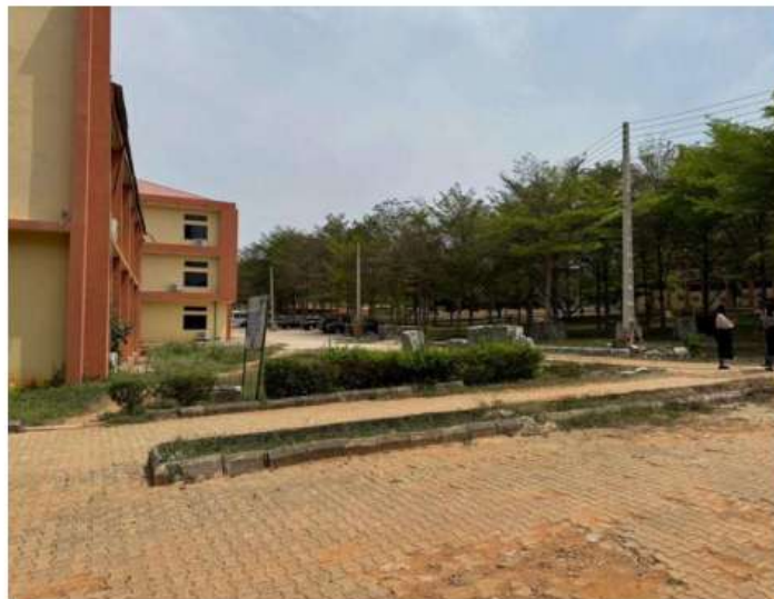
Plate 7: Academic court — paving terminating abruptly, large unpaved laterite zone, broken kerb edges
